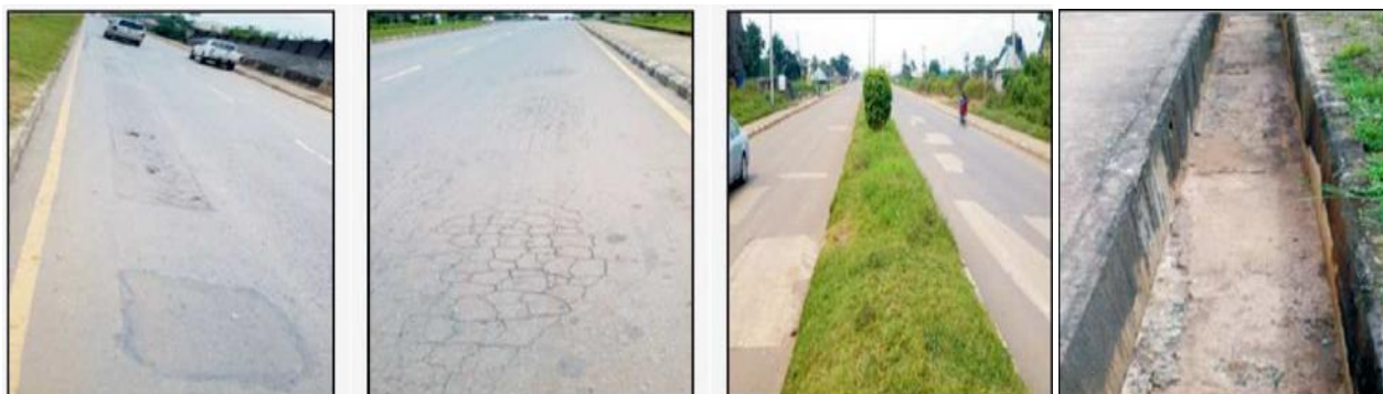
Figure 2 The Enugu - Abakaliki Road with potholes, ruts, alligator cracking, fatigue concrete & U-Shaped concrete drains (Source: Babadiya & Igwe 2021)
