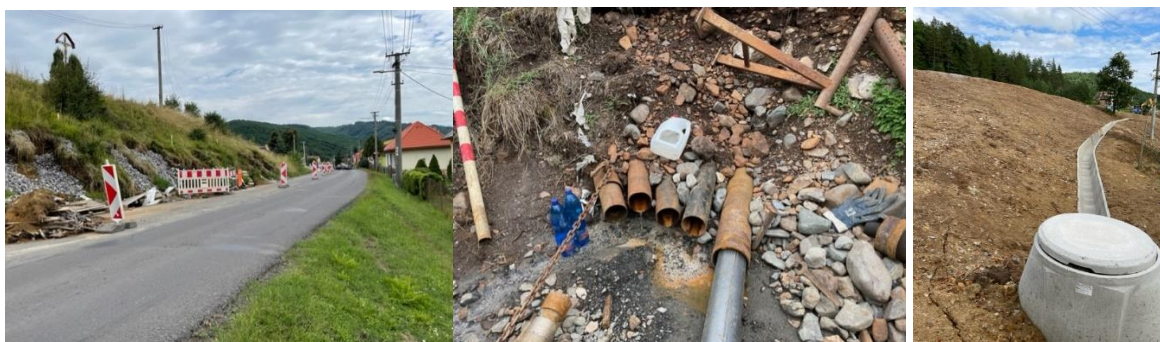
Figure 1. From left – outlet of prefabricated drains at the foot of the landslide; realization of horizontal drainage wells; surface rigol and control shaft
