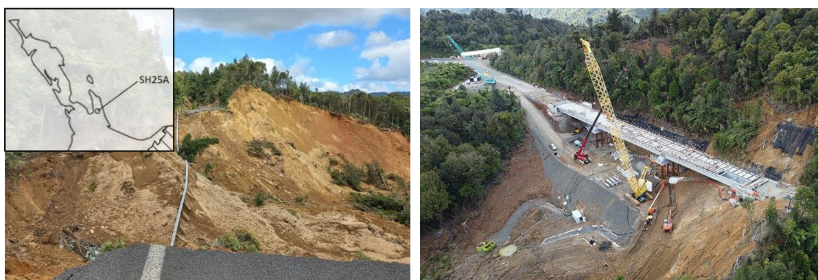
Figure 1. Upper left: landslide impacting SH25a. Upper right: bridge solution under construction (photograph from Waka Kotahi NZ Transport Agency)
