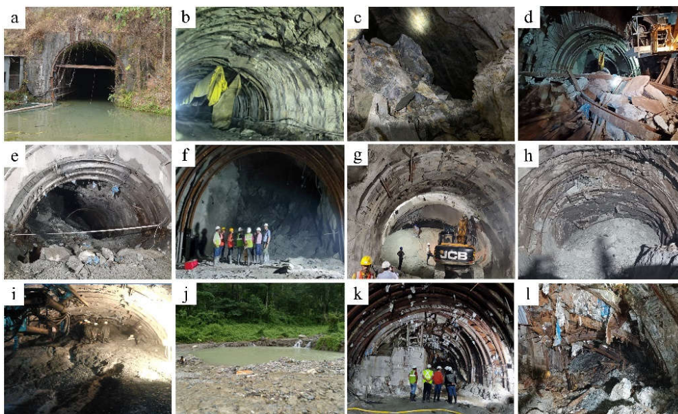
Figure 3. Showing Photographs of Hindrances faced during resumption of Underground works. (a) Water accumulation at Tunnels. (b) Twisting and Buckling in Lattice girder. (c) & (d) Rockfall and cavity formation in already excavated tunnel portion (e), (f), (g) & (h) huge cavities and collapsed tunnel area in already excavated tunnel portion. (i) & (j) Collapsed tunnel face and surface cave-in above the tunnel at Kalej Khola (k) & (l) Collapsed tunnel below Kamlet Khola.
