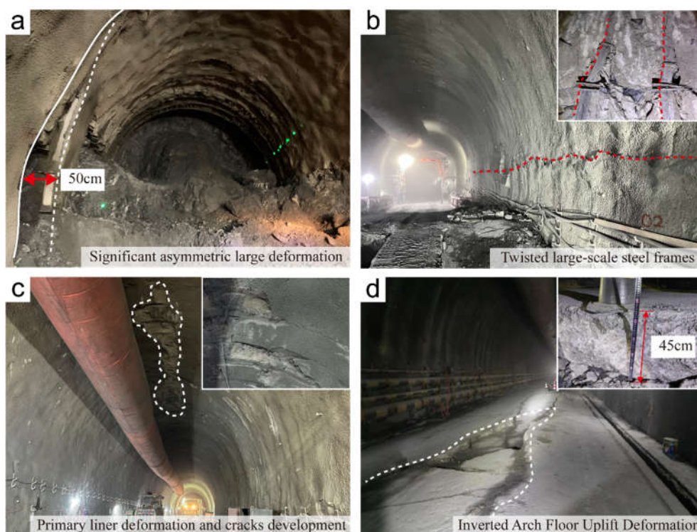
Figure 1. Large deformation and typical failure characteristics of supporting structure of tunnel project.
