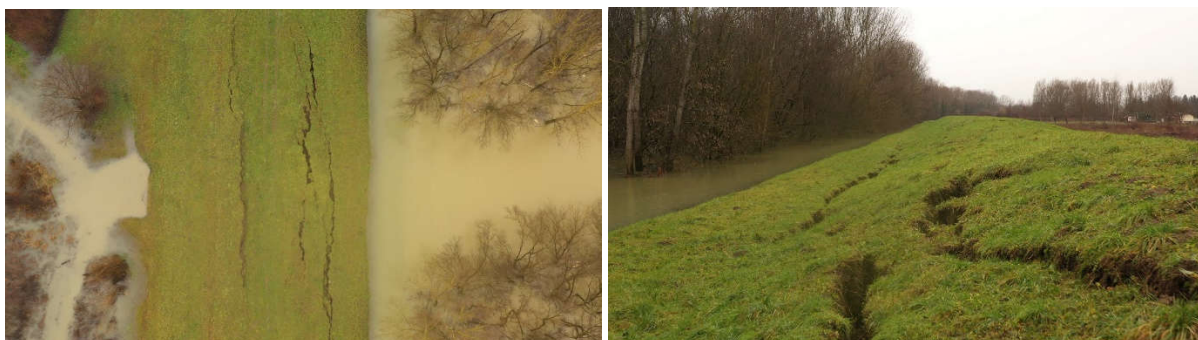
Figure 1. Deformed levees as a consequence of earthquake - induced liquefaction in Sisak – Moslavina County
