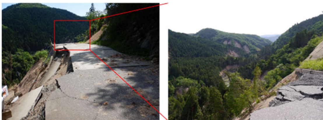
Figure 12. Image at Loc.VI. Collapse of a prefectural road.
