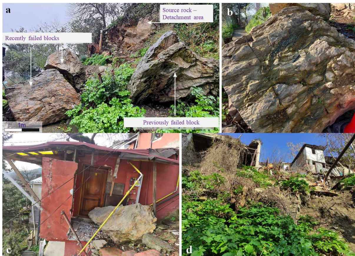
Figure 2. Views of a) failed blocks b) closer view of nodular limestone c) damaged building d) risky natural and man-made debris material.
