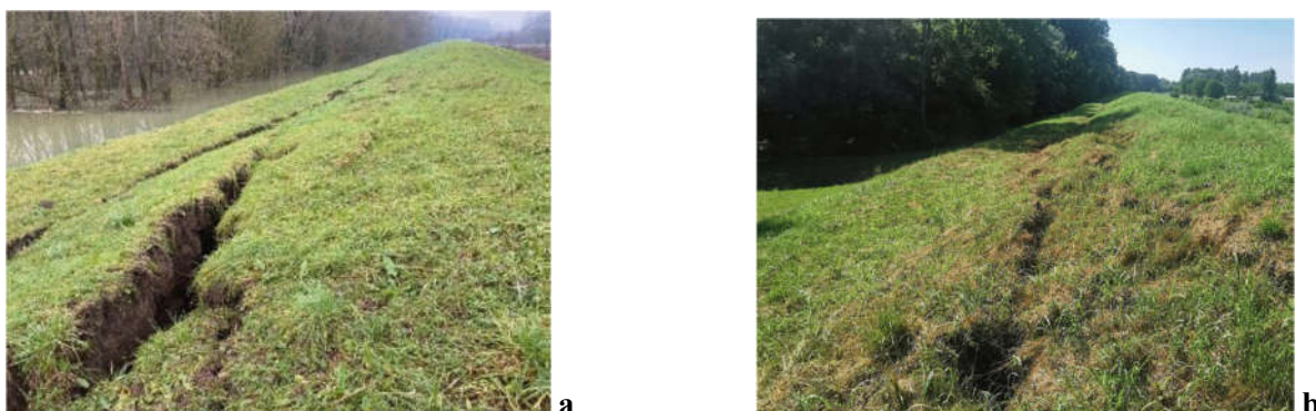
Figure 1. Comparison of the levee crack: a) immediately after the earthquake and b) after 6 months
