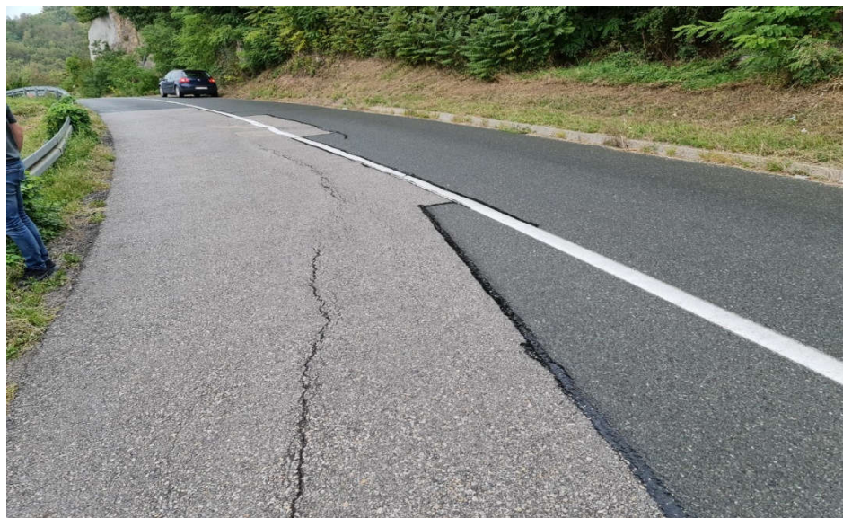
Figure 17. Western part of the road with developed crack about 15 meters long
