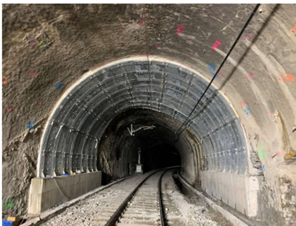
Figure 9. Situation at the end of the safety works (same point of view as Figure 1)
