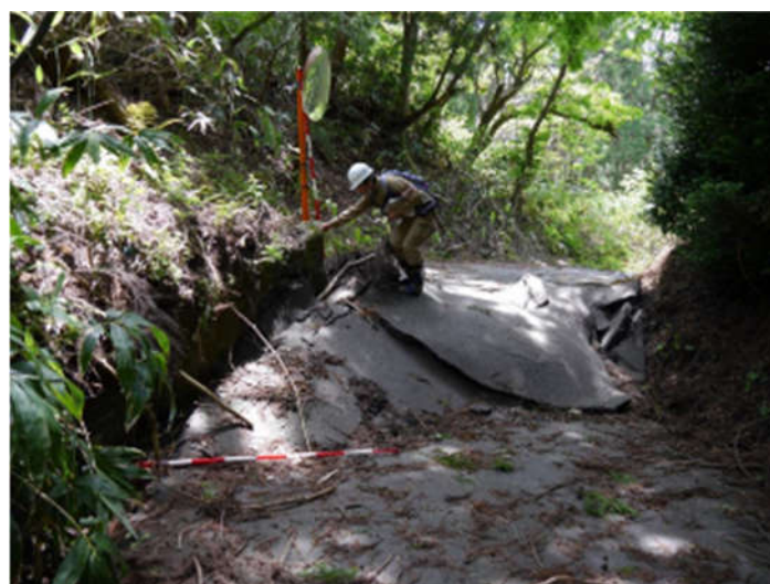
Figure 11. Image at Loc. V. Internal deformation of mobile unit, with 1.2 m longitudinal displacement and 1.6 m horizontal displacement on the right side.
