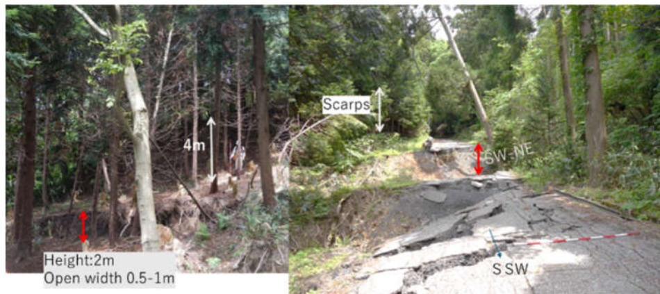
Figure 7. Image at Loc. I, showing the southward lowering of a step on the west side of Hattaro Pass, which occurred approximately 5 m in front of a small cliff topography (4 m high).
