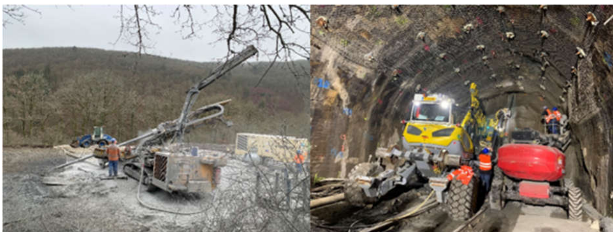
Figure 8. On the left: drilling from above to inject the grout. On the right: drilling from the tunnel for anchoring the deconsolidated soil injected above the hole in the vault
