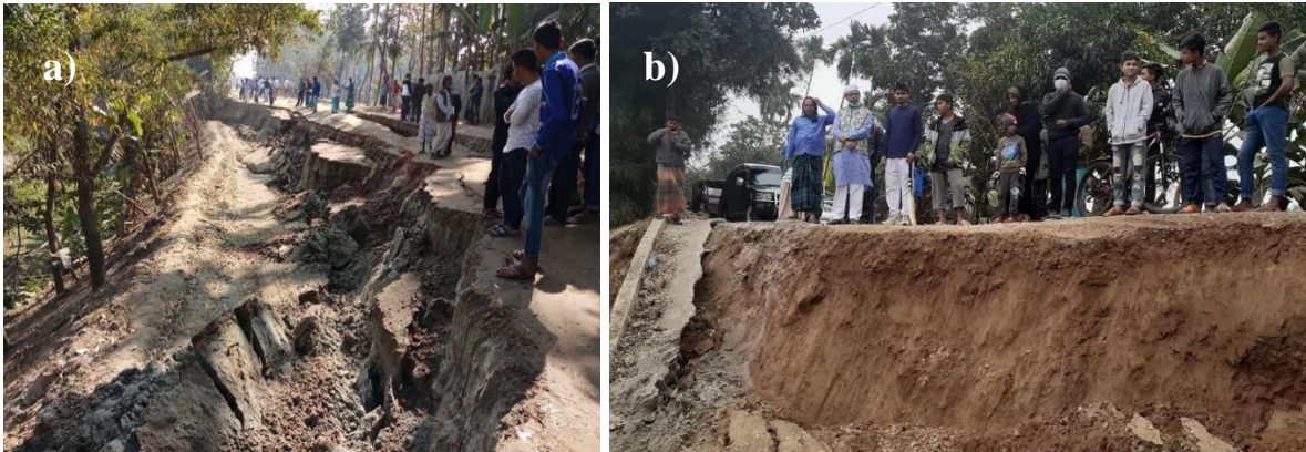
Figure 1 a) (Photo credit: The Daily Asian Age) Road collapse between Kapasia-Sreepur on 13 February 2018, b) (Photo credit: The Dhaka Tribune) Part of the Kapasia-Sreepur road collapsed in Kapasia Upazila of Gazipur District, December 11, 2020.
