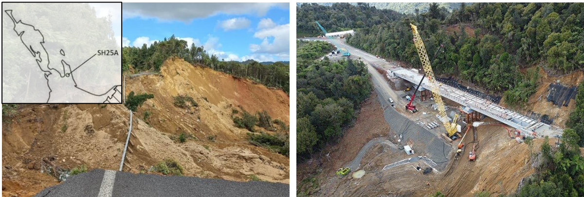
Figure 1. Upper left: landslide impacting SH25a. Upper right: bridge solution under construction (photograph from Waka Kotahi NZ Transport Agency)
