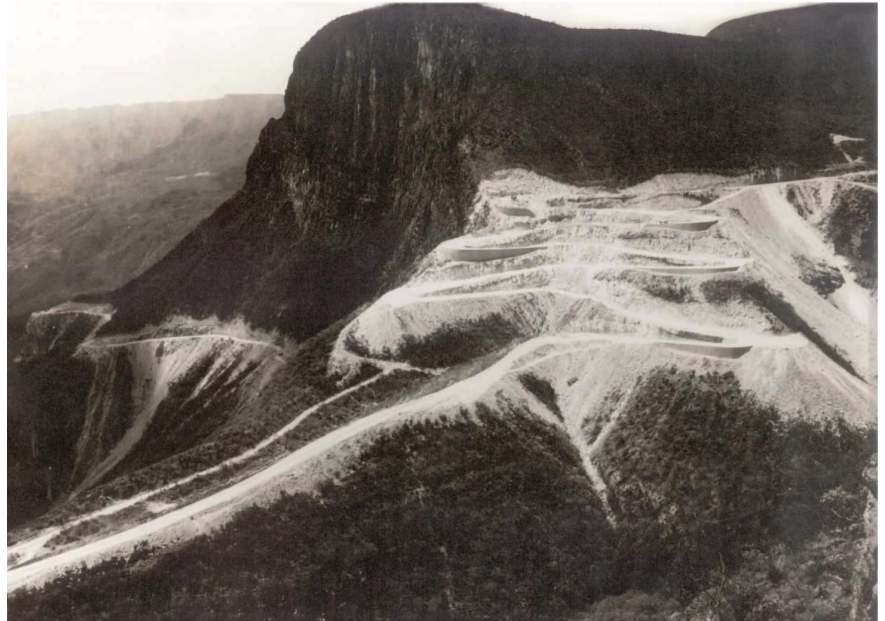
200 m descent with switchbacks. Road under construction through Serra da Leba (south of Angola) in early seventies. Excavated rocks were used to construct shallow masonry walls and after vegetation recolonised the earth works, the road became well integrated into the mountain landscape
