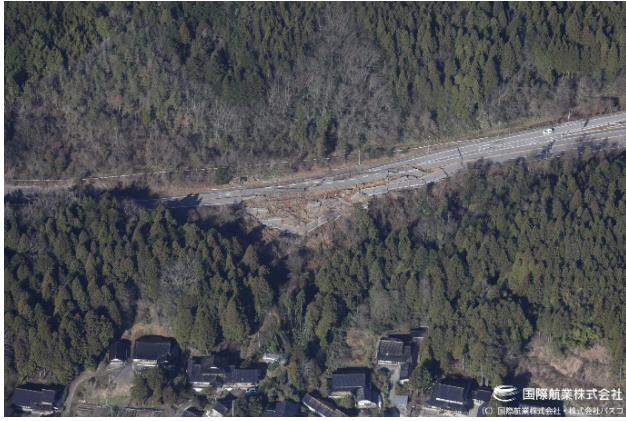
Fig. 6 Damage to the Noto Satoyama Kaido Road, that directly connects Kanazawa City to the Noto Peninsula, Ishikawa Prefecture
