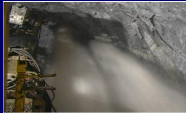
Tunnel Water Inrush
