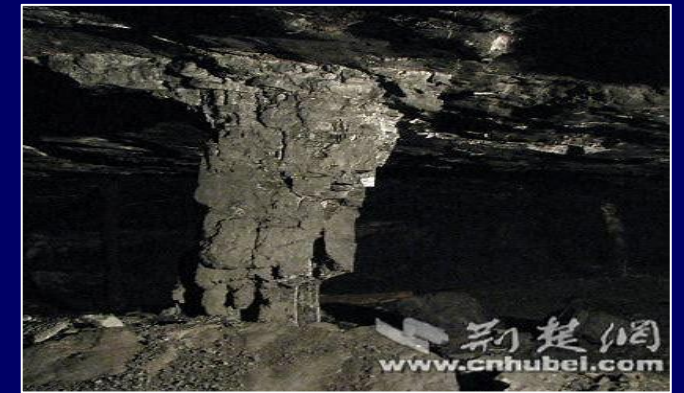
Mine Prop Failure
