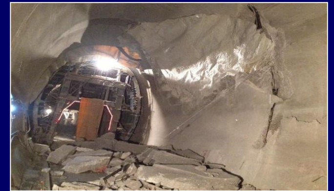
Tunnel Lining Failure
