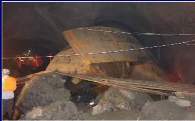
Tunnel Roof Collapse
