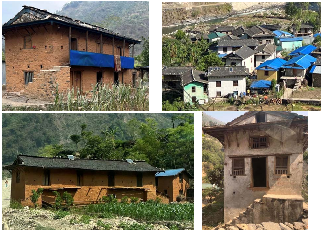
Figure 4, Rural buildings in Barekot and Nalgad municipalities of Jajarkot district (Photographs taken in June 2023)
