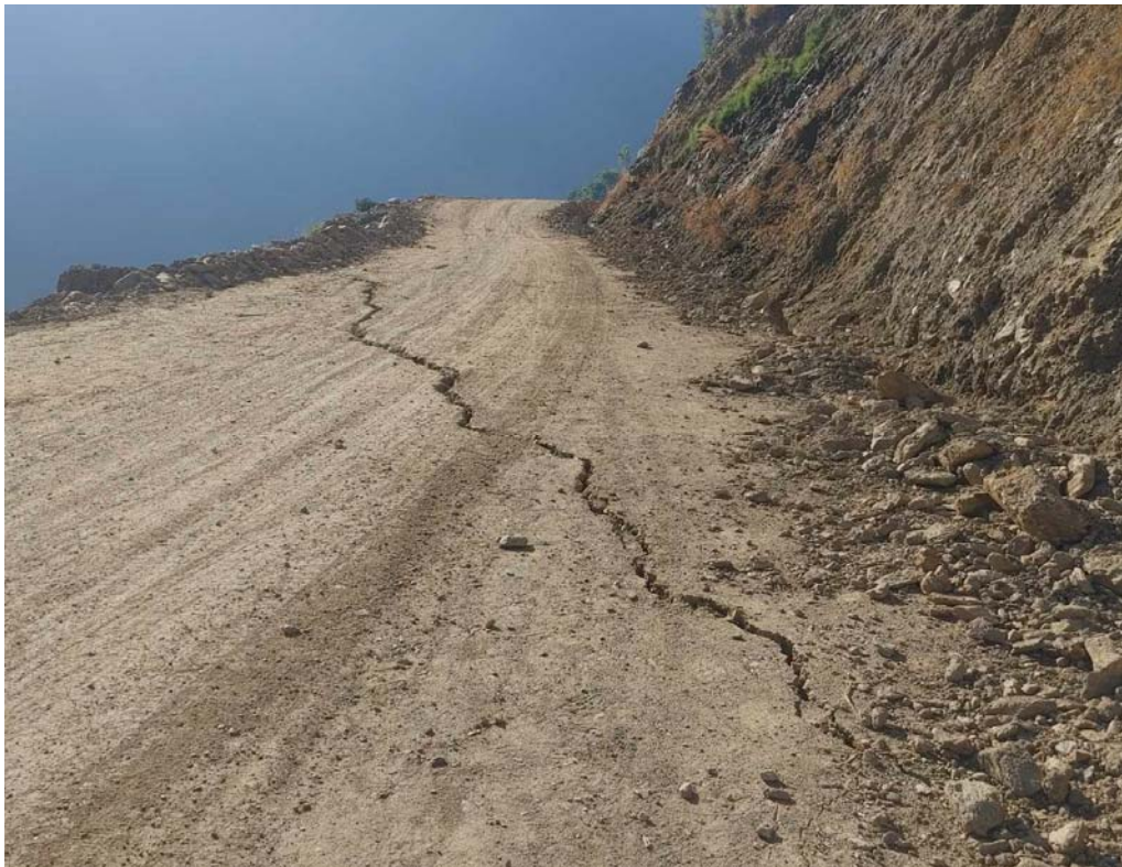
Figure 7, Typical cracks on road after the earthquake (source of top photo: RSS, Nepal and bottom photo: Dr. Lok Bijaya Adhikari)
