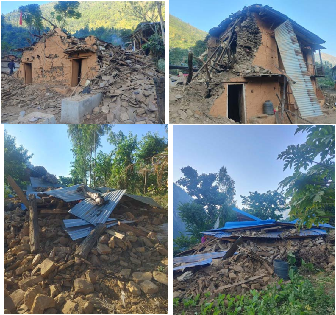
Figure 6, Typically damage pattern of mud mortar type buildings in Nalgad Municipality, Jajarkot district (Photo: Dr. Lok Bijaya Adhikari)
