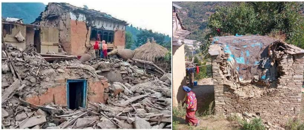
Figure 5, Typical rural building damages after the earthquake (Photo: Manju Joshi)
