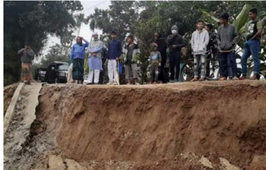
Figure 2: Part of the Kapasia-Sreepur road collapsed in Kapasia Upazila of Gazipur District, December 11, 2020, Photo credit: The Dhaka Tribune
