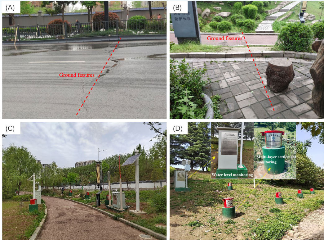
Fig. 7 Ground fissure and layerwise mark (the location of A, B, C and D is shown in Fig. 6)
